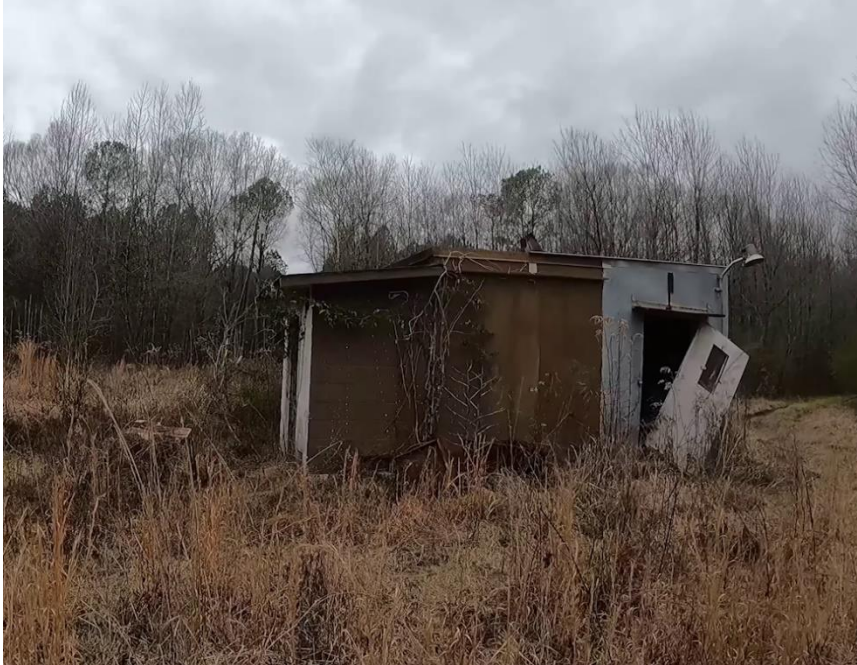
WJLX AM transmitter site after the alleged theft. Tower pedestal to the left of the building. (William Collier)
