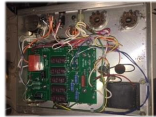
Fig 9 New board wired in and wires dressed
