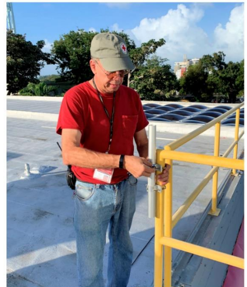
Puerto Rico Section Manager Oscar Resto, KP4RF, installs an antenna at Red Cross Headquarters in San Juan.
